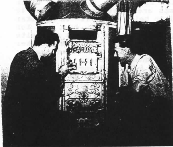
The author (left) and an serviceman check out a furnace prior to installing a stoker
